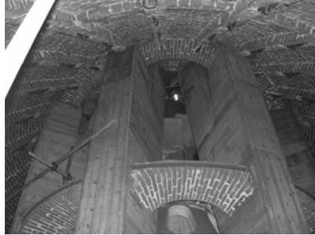
Fig. 1 (left). View of the double order of Corinthian columns of the dome and lantern
