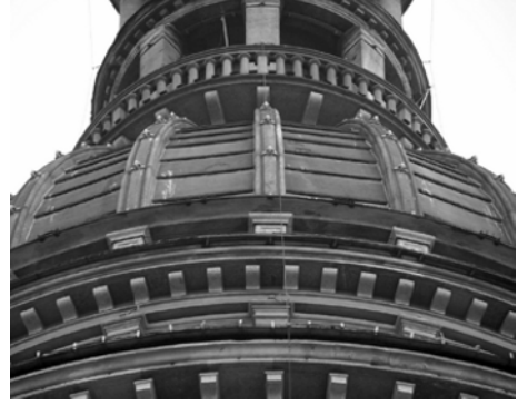
Fig.13. External covering: dados and restraining rings of the finishing in correspondence with the internal rib system
