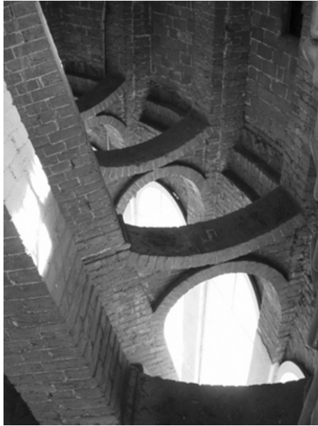
Fig. 11. View of the upside-down stiffening arches
