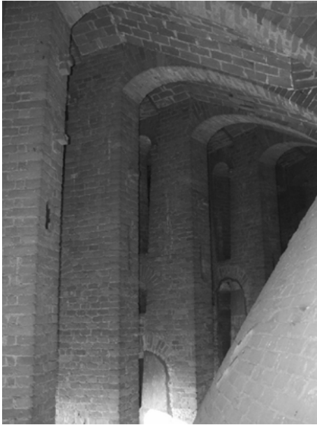
Fig. 10. system of climbing arches that support the catwalk above the interior dome
